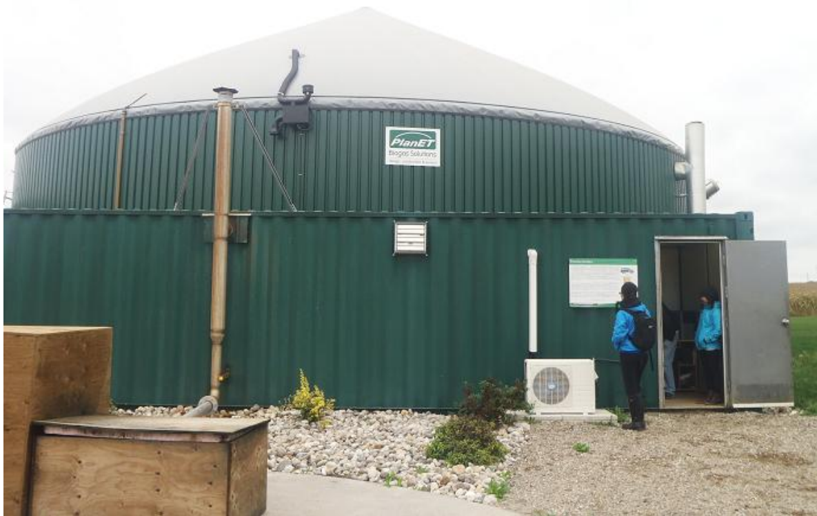
Figure 9. Biogas Facility from Ledgecroft Farm, Ontario
